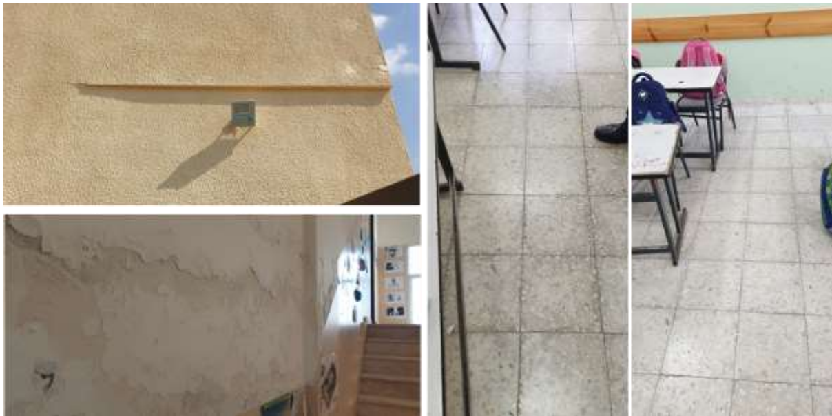
Figure 4 Eccentric wall and water damage at Jubara school (left) and tiles deficiencies at Al Manshiya school (Right)
