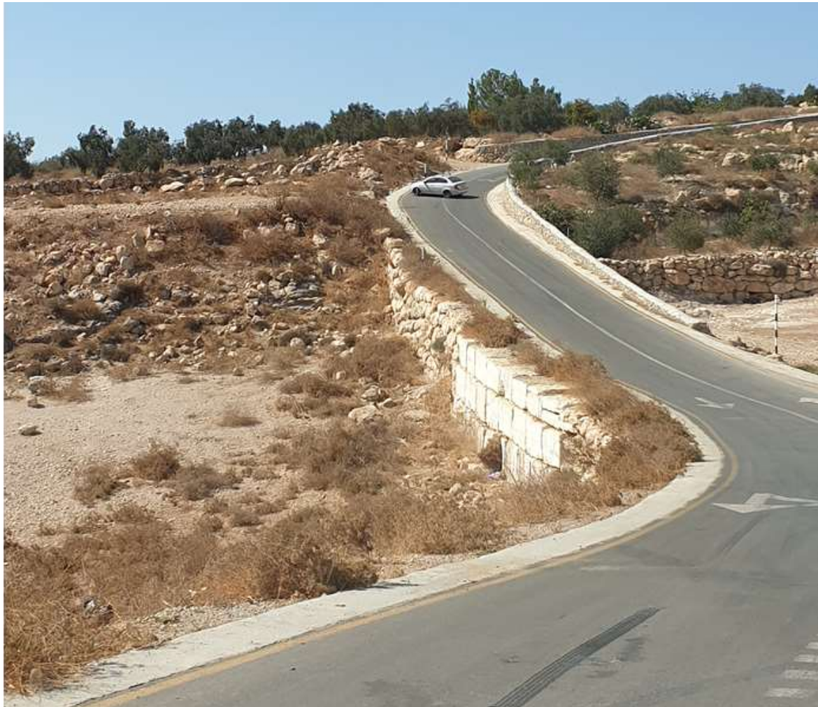
Figure 3 Idna road - limited sight distance curve (left) and major watercourse without culvert (right)
