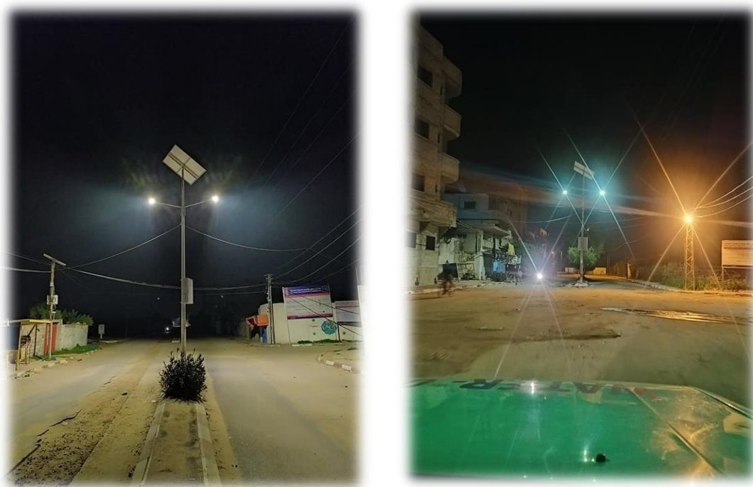
Figure 11: Streetlights at Abasan Al Jadeda during night
